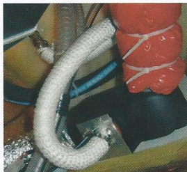
The exhaust swan neck is high enough to reduce the chances of sea water getting into the heater
