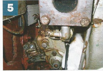
5 The underside. The exhaust manifold is warped, the Mirimax injector pump leaks oil from the feed pipe unions and way down below is the remains of both the mechanical fuel lift pump and the main oil filter – plus the engine controls
