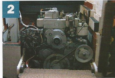
2 The old Albin in all its glory – remove the engine box and local furniture to give you as much space around the engine as possible
