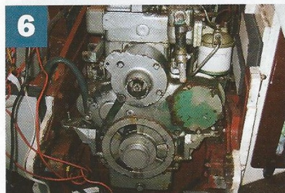
6 Remove the water pump, exhaust tail pipe, alternator and fuel filter to be able to get at the engine mounting bolts. With the alternator out the wood can be seen for the trees. One of the forward fixing studs can be got at, but before then the wiring needs sorting. Tag and name each wire before you disconnect as it saves hours of worry and testing afterwards. The engine intake heater (the plug and pipe in the air intake casing) also needs removing
